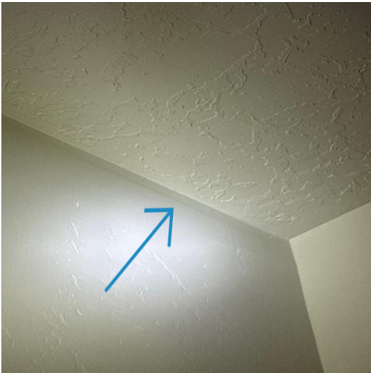
Image Number: 27 Observation: Discoloration was observed at the drywall indicating possible moisture intrusion.
