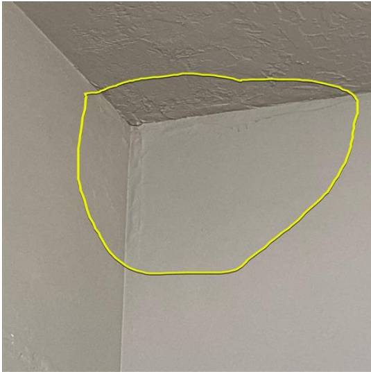
Image Number: 7 Observation: Observation: Bubbling paint and moisture staining were observed, indicating active or prior moisture intrusion from above.
