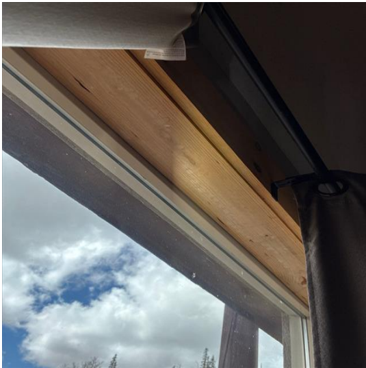
Image Number: 42 Observation: Observation: Water staining was observed at the window jamb extensions in all the rooms. Possible sources include moisture intrusion from the roof system above, window flashing or sealant failure, or condensation. A definitive source could not be determined from visual inspection alone.
