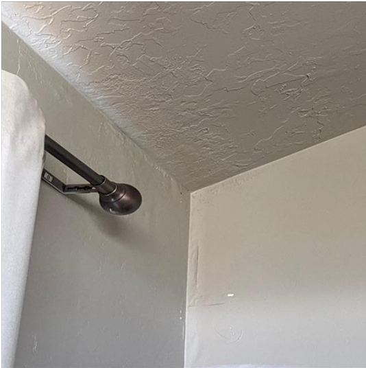
Image Number: 11 Observation: Bubbling paint and moisture staining were observed, indicating active or prior moisture intrusion from above.
