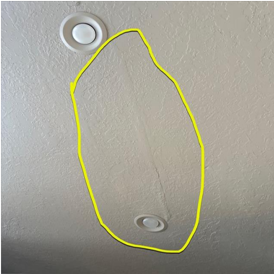
Image Number: 25 Observation: Peeling tape and bubbled paint were observed in the kitchen indicating possible moisture intrusion.
