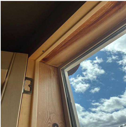
Image Number: 41 Observation: Observation: Water staining was observed at the window jamb extensions in all the rooms. Possible sources include moisture intrusion from the roof system above, window flashing or sealant failure, or condensation. A definitive source could not be determined from visual inspection alone.
