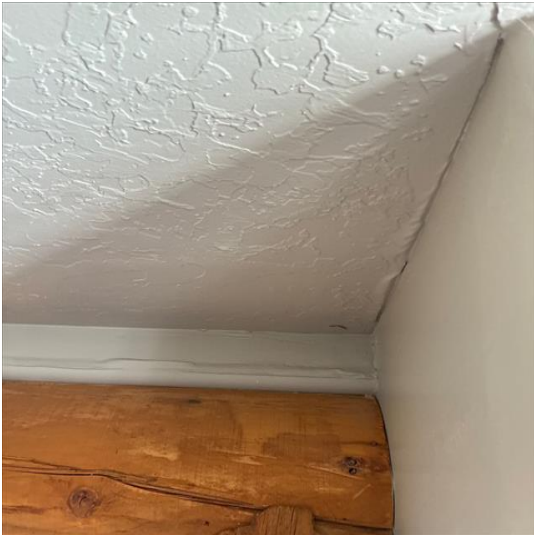
Image Number: 34 Observation: Bubbling paint was observed at the ceiling near the roof pitch transition.
