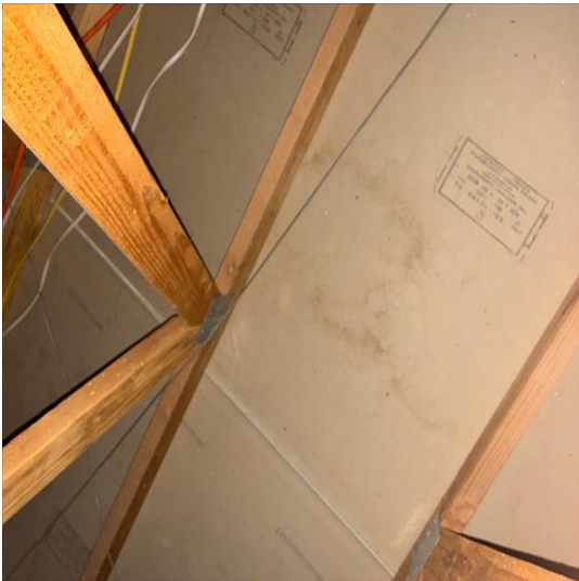
Image Number: 84 Observation: Observation: Garage: Moisture stains were noticed along the eaves and valley rafters. Moisture stains were noticed on the garage drywall as well indicating roof leak. Roof access was limited and was unable to pinpoint where all the locations are.
