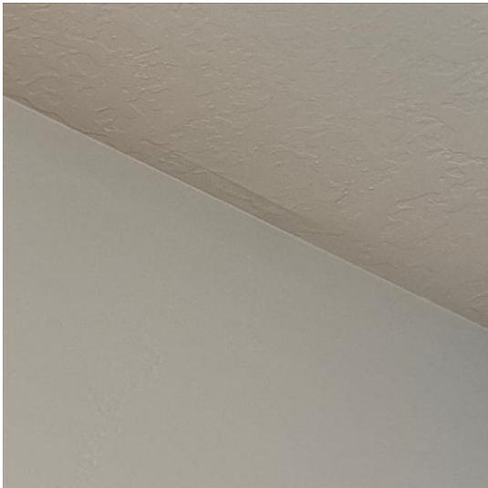
Image Number: 9 Observation: Observation: Cracking in the drywall sealing was observed.
