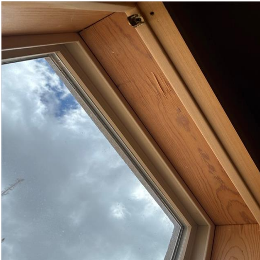
Image Number: 48 Observation: Observation: Water staining was observed at the window jamb extensions in all the rooms. Possible sources include moisture intrusion from the roof system above, window flashing or sealant failure, or condensation. A definitive source could not be determined from visual inspection alone.
