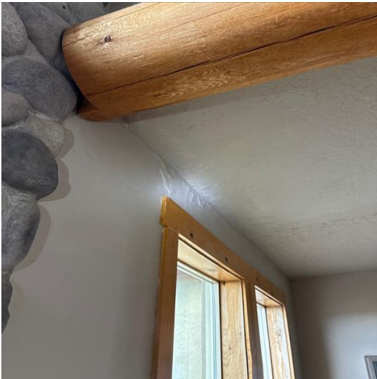
Image Number: 18 Observation: The upper drywall was repaired from the ice dam, and the paint is showing signs of moisture intrusion.
