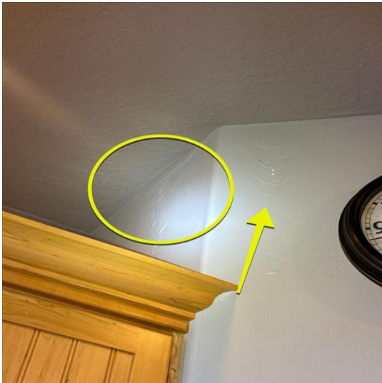
Image Number: 24 Observation: Observation: Peeling tape and bubbled paint were observed in the kitchen indicating possible moisture intrusion .
