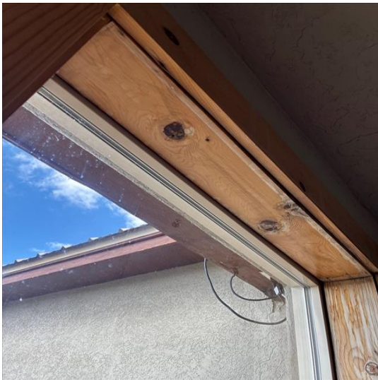
Image Number: 47 Observation: Observation: Water staining was observed at the window jamb extensions in all the rooms. Possible sources include moisture intrusion from the roof system above, window flashing or sealant failure, or condensation. A definitive source could not be determined from visual inspection alone.
