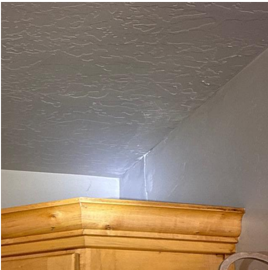
Image Number: 35 Observation: Bubbling paint was observed at the ceiling near the roof pitch transition.
