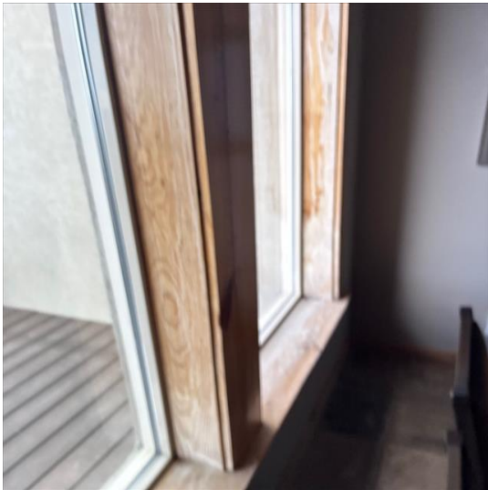
Image Number: 45 Observation: Observation: Water staining was observed at the window jamb extensions in all the rooms. Possible sources include moisture intrusion from the roof system above, window flashing or sealant failure, or condensation. A definitive source could not be determined from visual inspection alone.
