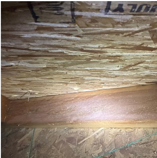
Image Number: 80 Observation: Observation: Garage: Moisture stains were noticed along the eaves and valley rafters. Moisture stains were noticed on the garage drywall as well indicating roof leak. Roof access was limited and was unable to pinpoint where all the locations are.
