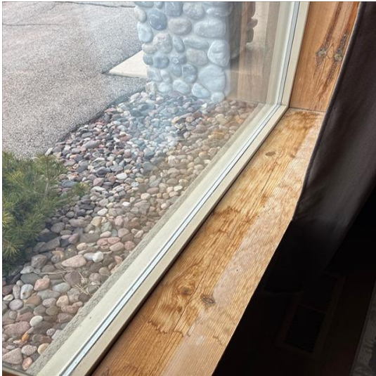
Image Number: 43 Observation: Observation: Water staining was observed at the window jamb extensions in all the rooms. Possible sources include moisture intrusion from the roof system above, window flashing or sealant failure, or condensation. A definitive source could not be determined from visual inspection alone.
