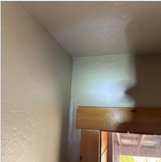
Image Number: 33 Observation: Observation: Bubbling paint was observed at the ceiling near the roof pitch transition.
