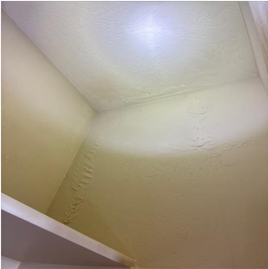
Image Number: 31 Observation: Observation: Living room closet. There are some discoloration and bubbling of the paint indicating moisture intrusion.
