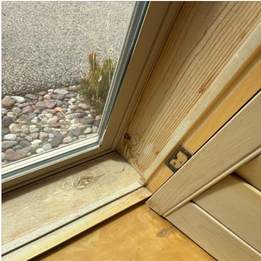
Image Number: 40 Observation: Observation: Water staining was observed at the window jamb extensions in all the rooms. Possible sources include moisture intrusion from the roof system above, window flashing or sealant failure, or condensation. A definitive source could not be determined from visual inspection alone.
