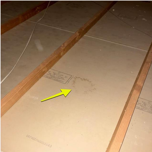
Image Number: 83 Observation: Observation: Garage: Moisture stains were noticed along the eaves and valley rafters. Moisture stains were noticed on the garage drywall as well indicating roof leak. Roof access was limited and was unable to pinpoint where all the locations are.
