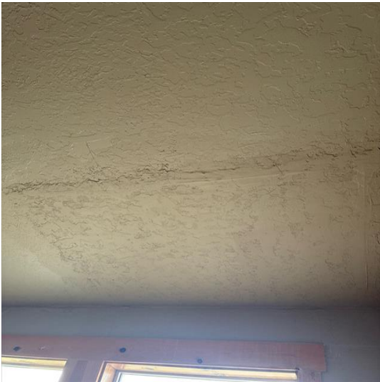
Image Number: 17 Observation: This is a previous drywall repair due to an ice dam 2-3 years ago. A roof repair seems to have been done, alongside an installed heat cable.
