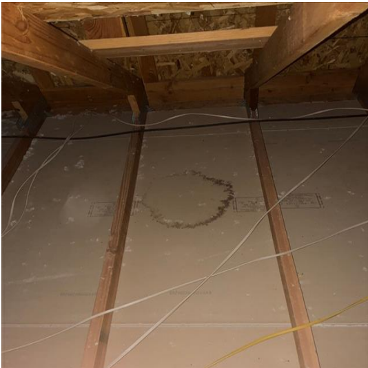
Image Number: 78 Observation: Observation: Garage: Moisture stains were noticed along the eaves and valley rafters. Moisture stains were noticed on the garage drywall as well indicating roof leak. Roof access was limited and was unable to pinpoint where all the locations are.
