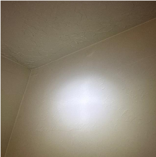
Image Number: 16 Observation: Bubbling paint and moisture staining were observed, indicating active or prior moisture intrusion from above.
