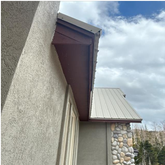
Image Number: 99 Observation: Soffit overview. ** No intake ventilation was observed during this inspection. This is important to have a proper ventilated home. Remedy: Install soffit ventilation according to proper NFA guidelines.
