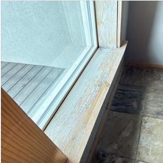
Image Number: 46 Observation: Observation: Water staining was observed at the window jamb extensions in all the rooms. Possible sources include moisture intrusion from the roof system above, window flashing or sealant failure, or condensation. A definitive source could not be determined from visual inspection alone.
