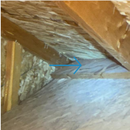
Image Number: 79 Observation: Observation: Garage: Moisture stains were noticed along the eaves and valley rafters. Moisture stains were noticed on the garage drywall as well indicating roof leak. Roof access was limited and was unable to pinpoint where all the locations are.
