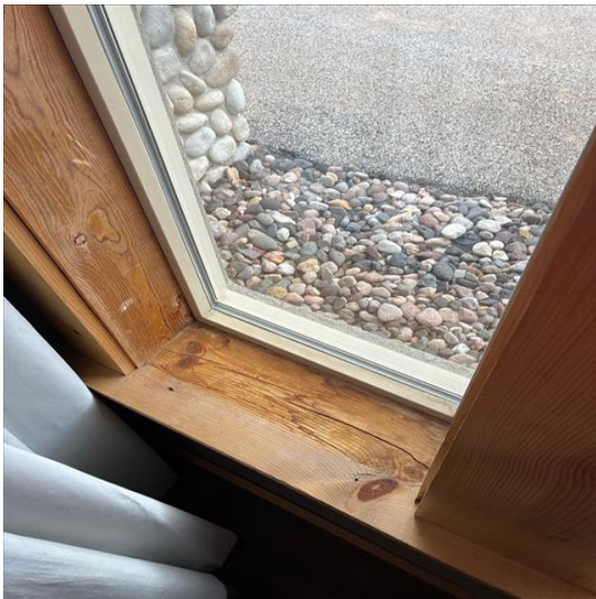
Image Number: 44 Observation: Observation: Water staining was observed at the window jamb extensions in all the rooms. Possible sources include moisture intrusion from the roof system above, window flashing or sealant failure, or condensation. A definitive source could not be determined from visual inspection alone.
